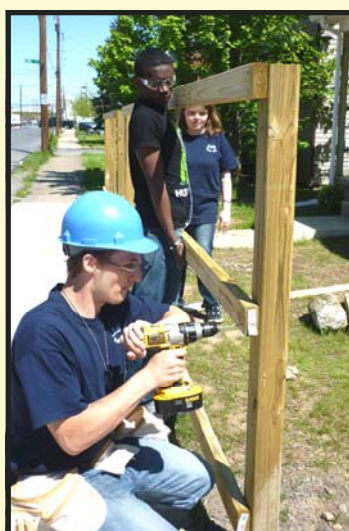
YouthBuild member, Todd Brown, gains hands-on experience as he constructs a perimeter fence at a Habitat for Humanity home in Williamsport.
